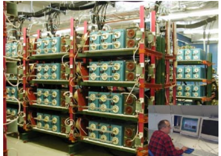
Figure 2: Pulsed power capacitor room and controls console
